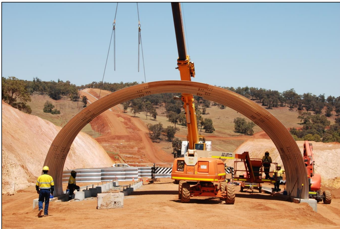
Trafficable Tunnel 442L – Worsley Efficiency & Growth project, Marradong Mine site, WA – during construction
