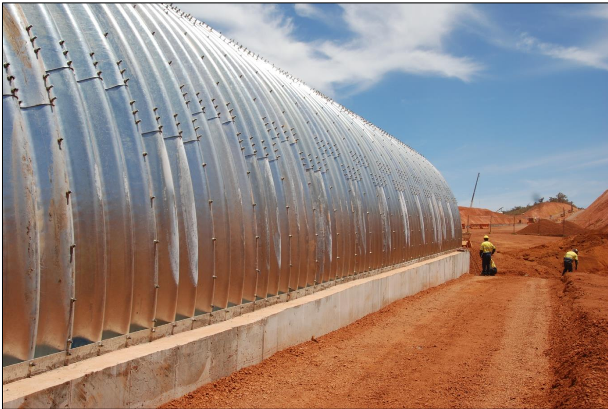
Trafficable Tunnel 442T – Worsley Efficiency & Growth project, Marradong Mine site, WA – during construction
