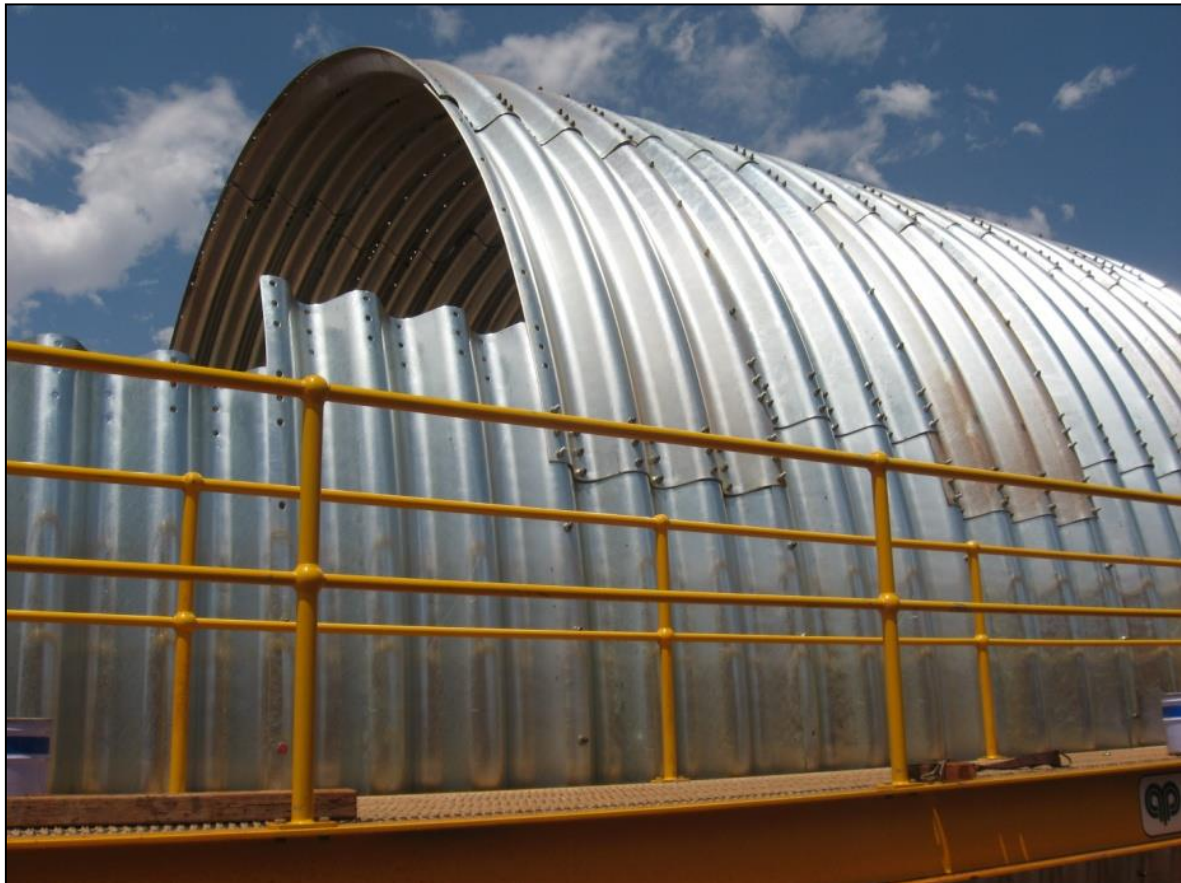
Duplicate large – span arch at Hamersley Iron / Rio Tinto's Yandi Mine site, WA – during construction
