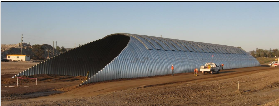
Large – span arch at Gibihi Road, Moura, Qld, AngloAmerican Coal, Dawson Mine site – during construction
