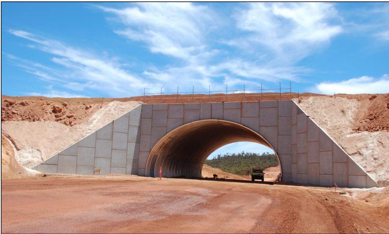
Trafficable Tunnel 442Q – Worsley Efficiency & Growth project, Marradong Mine site, WA – during construction
