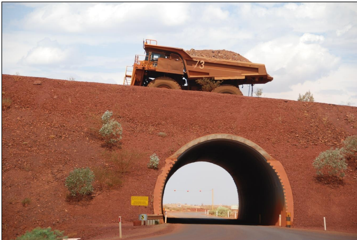
Large – span arch at Hamersley Iron / Rio Tinto’s Yandi Mine site, WA.
