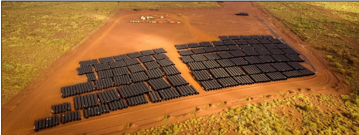
On-site manufacturing & culvert lay-down area at Gudai-Darri, Rio Tinto, the Pilbara, WA
